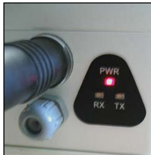
Figure 2. MET Station LEDs (Power –ON)
